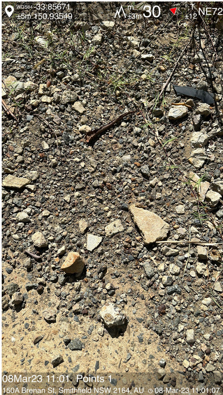
Plate 49: Example of potential ACM observed on the surface of 150a Brenan Street.
