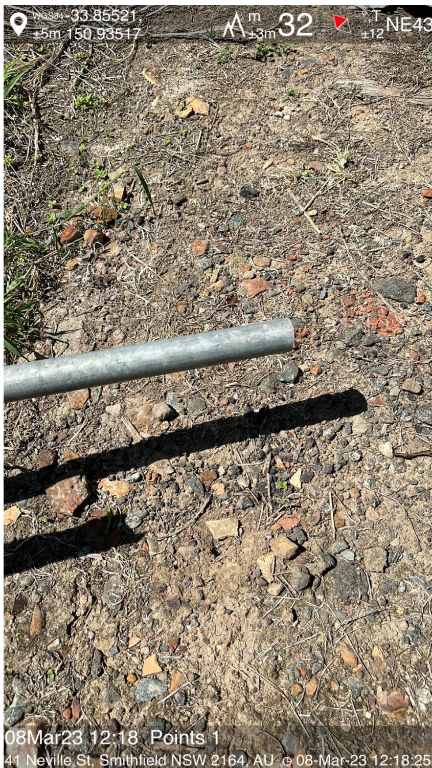
Plate 32: Example of potential ACM at the rear of No. 41 Neville Street.
